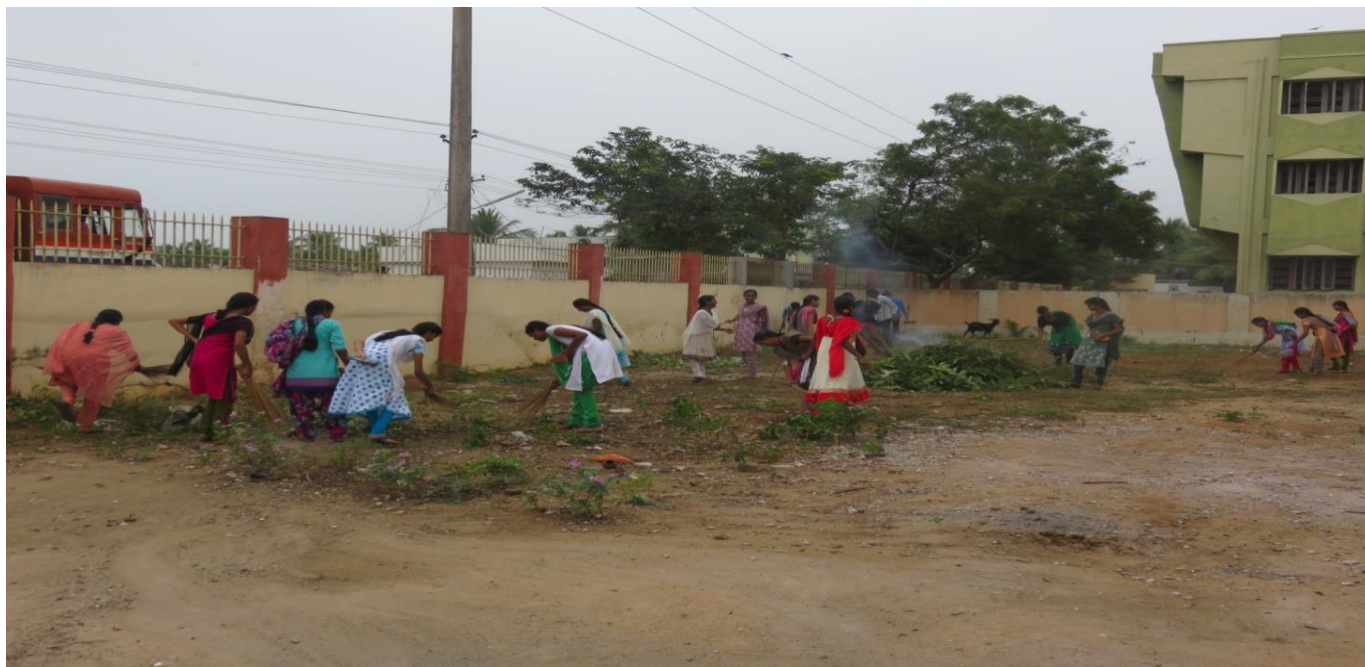
NSS Volunteers clearing bushes at Primary Health Center, Farampeta – an adopted village of NSS unit of Dr.S.R.K.Govt.Arts College, Yanam during Special Camp 22 nd - 28 th January, 2016.
